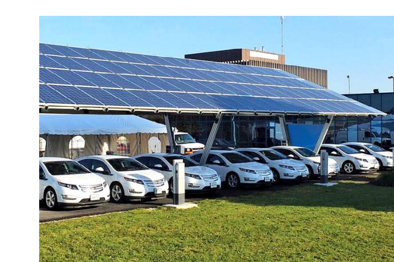
Figure 3. A solar-powered charging station.
